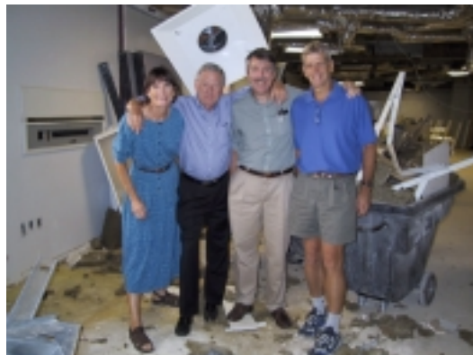
9/00: Susie Mumby, Al Gilman, Paul Sternweis, and Marc Mumby start the demolition.
